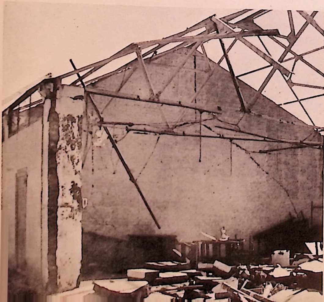
Roofs were the big victims, but even walls in places collapsed before the wind's fury. This was a school building.
