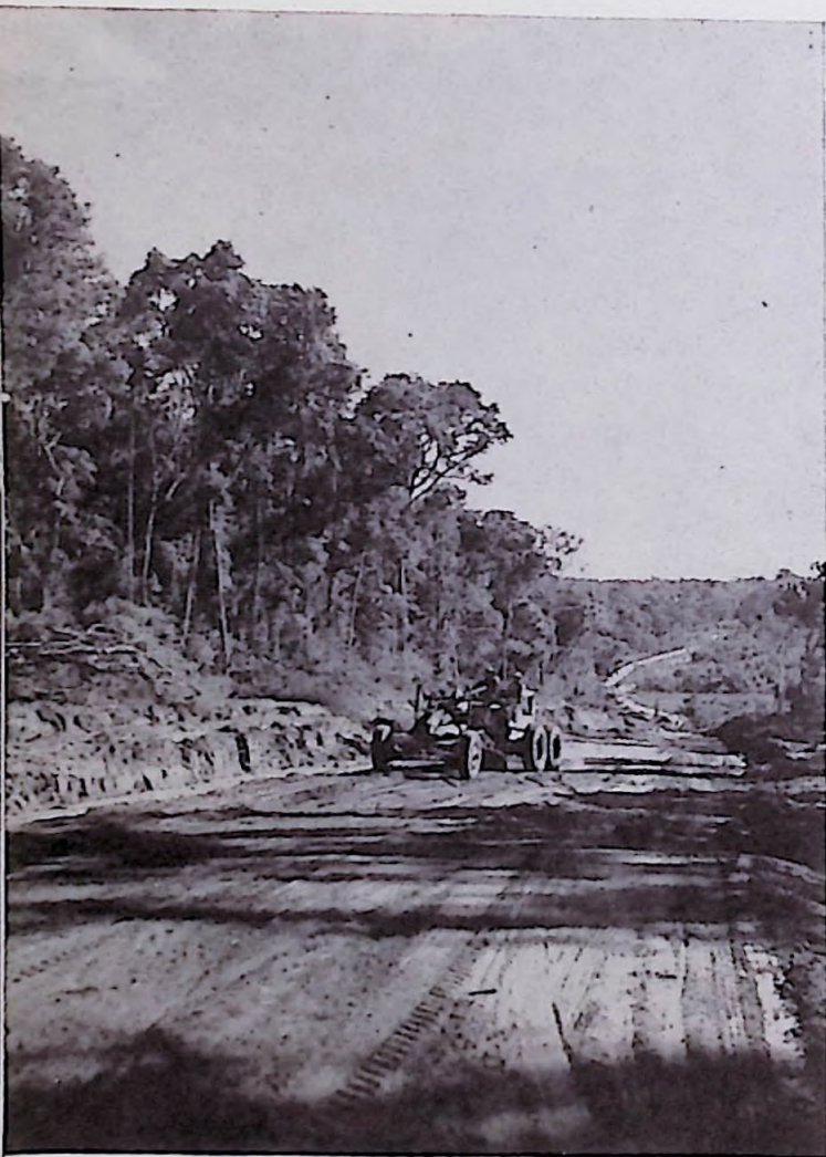
New highway under construction between the Parana River and Asuncion will be patrolled by ghosts of world's "First Christian State."
