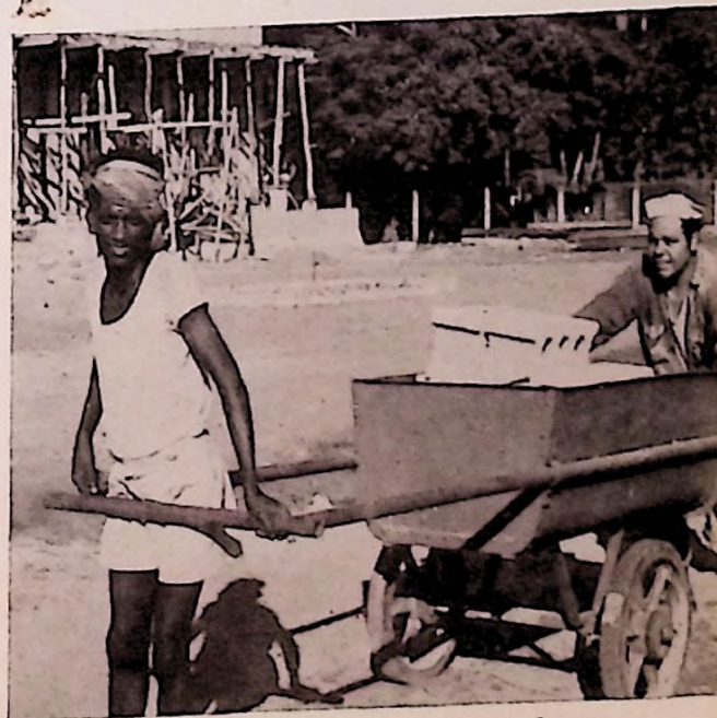
Brother Emmanuel Trujillo of New Orleans helping to build a school in Trincomalee.
