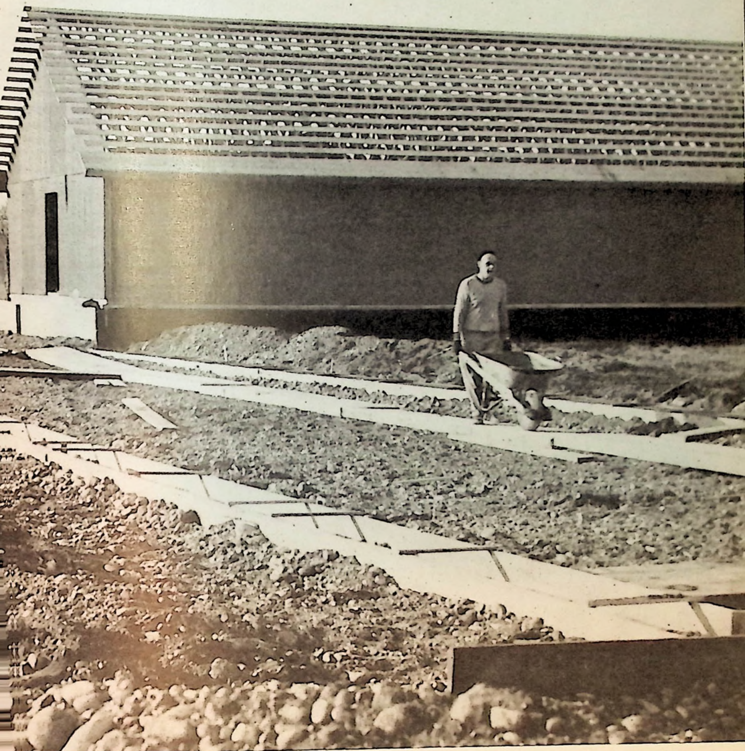
This girls dormitory, now completed, reveals the sturdy construction which is typical of all the buildings being erected at Copper Valley.
