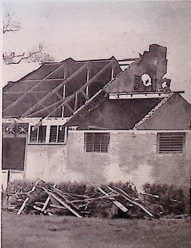
Part of the boarding school at St. George's College in Kingston, revealing damage to the roof.
