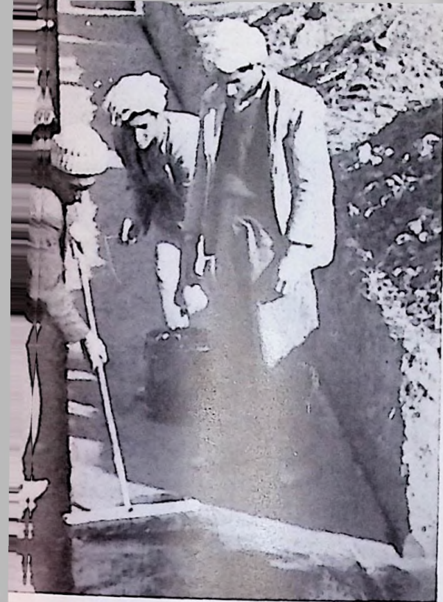
Mauroff, the only coadjutor brother on the mission, is the laying of the cement.
