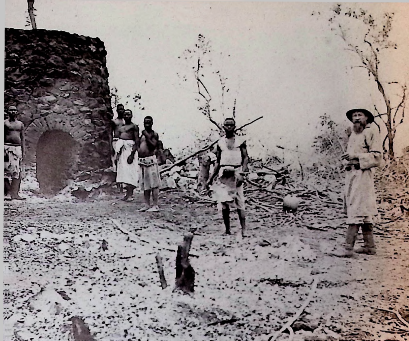
In Central Africa a White Father shows some of his African charges how to bake bricks for the new mission buildings.
