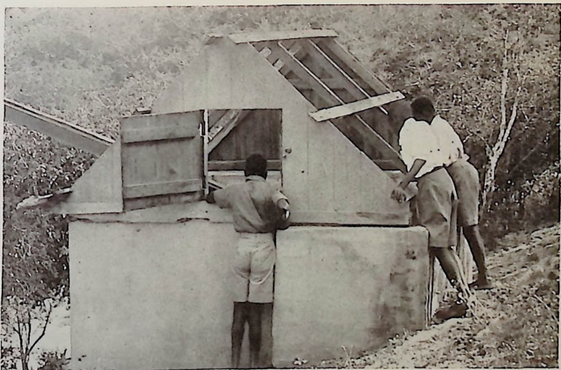
Port Henderson's very unreliable water tank and some of Father Owens' school boys seeing how empty it is.
