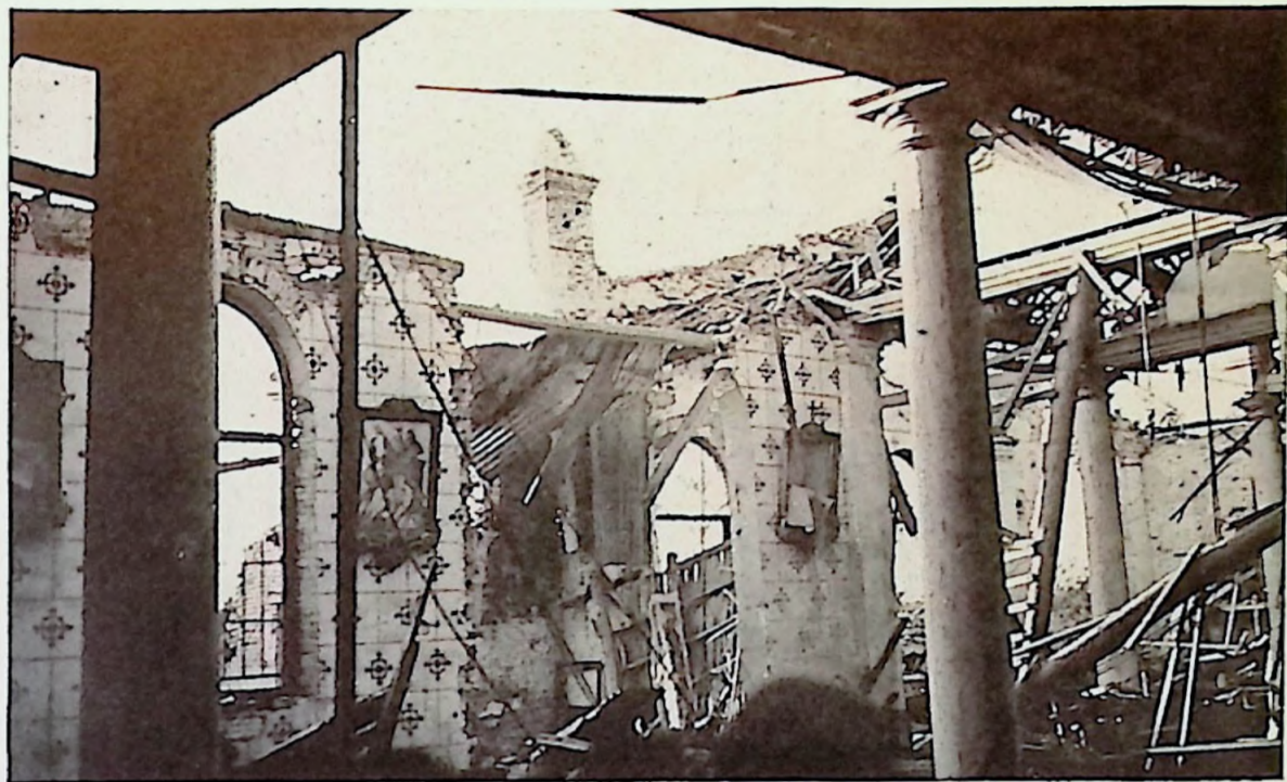
What the war did to the church of Tsangkalou. Father O'Hara reports that it is now almost completely restored.
