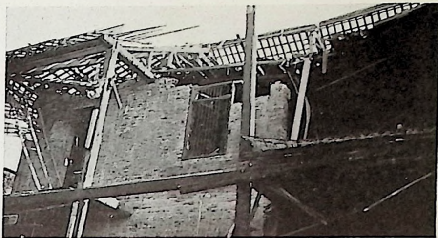
Damage wrought by a Japanese bomb which struck the roof of Ricci College conducted by the Jesuits at Nanking.
