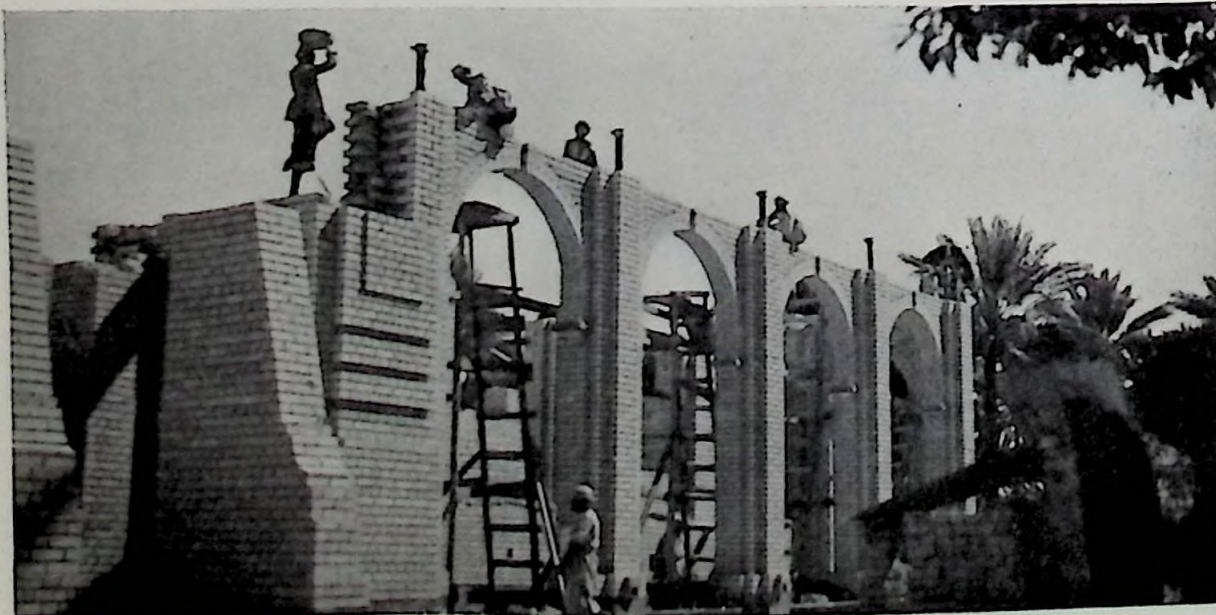
Workmen putting up the cloister arches in the new Baghdad College recently completed.
