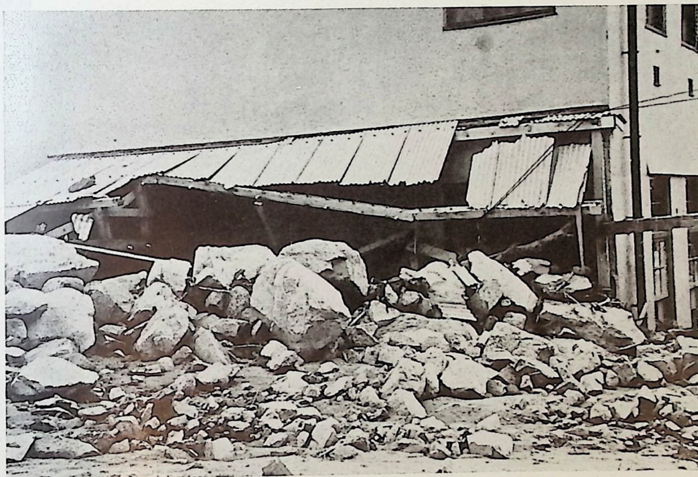
The north wall which received the full force of the flood. Huge boulders crashed through, filling classrooms and corridors.
