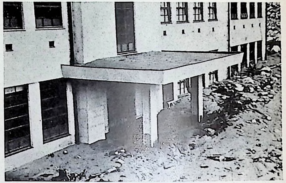
Front entrance of the new school after the landslide. Debris is piled up over the first story.
