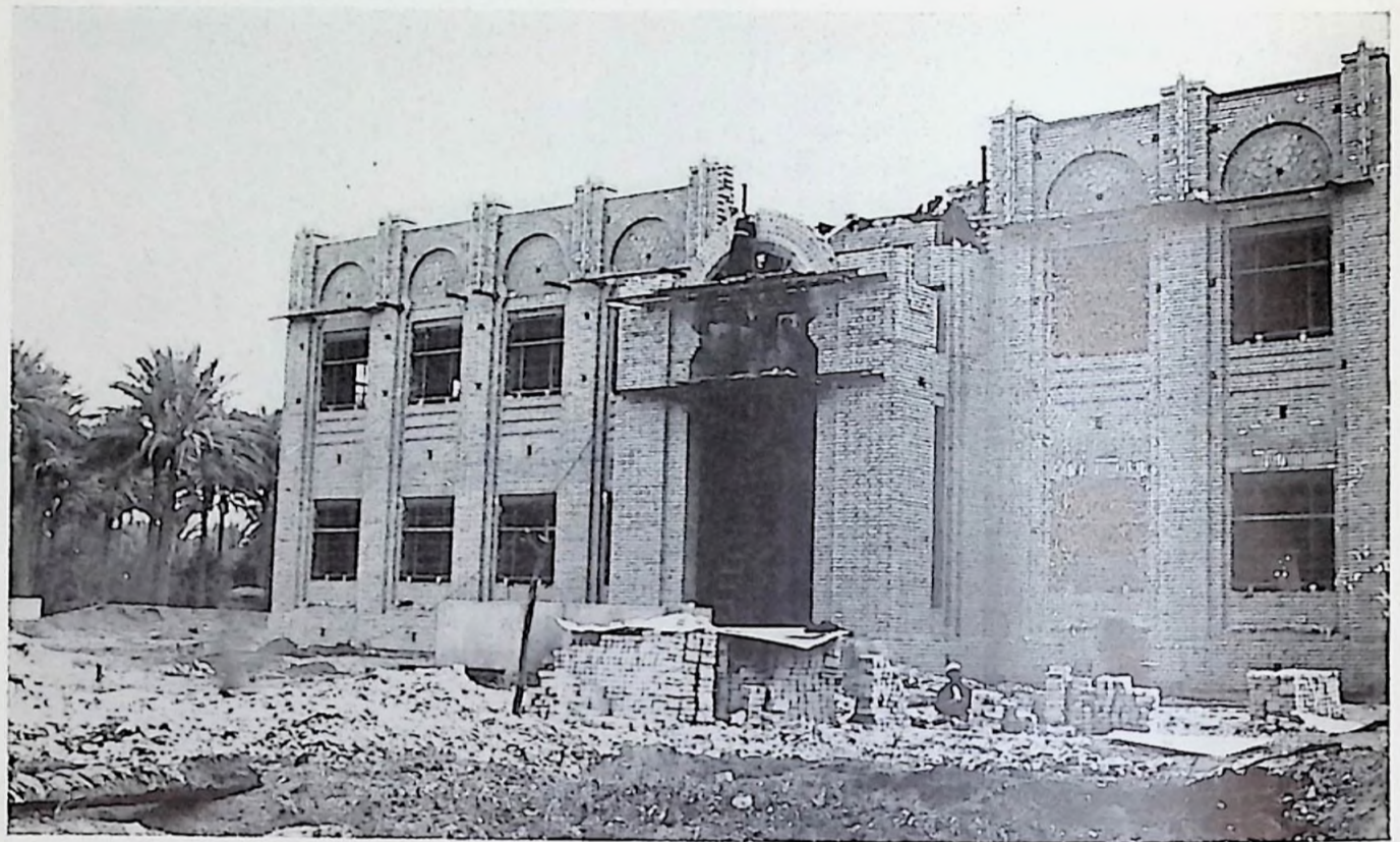
The central arch just over the entrance of the new Baghdad College in process of completion as of December, 1937.
