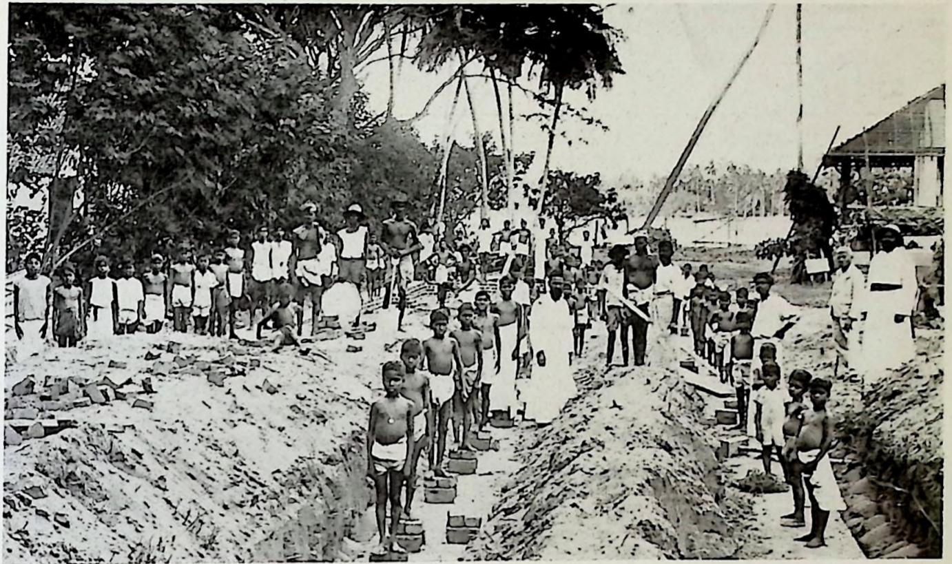
Putting down the foundations for a new school. Father Theophilus is his own contractor and every boy does his share of work.
