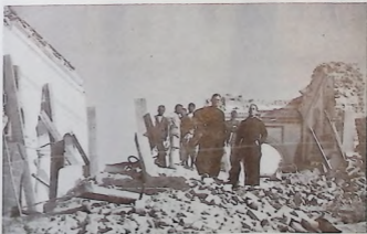
After the earthquake of January 15, 1934, Father Edward J. O'Leary, S.J. (left), Pastor of the church at Bettiah, and Vincent G. McGlinchy, S.J., standing on the ruins of what was Patna Mission's oldest church.
