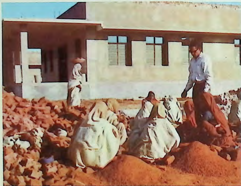
Br George Cheruparambill, S.J., directing work on the construction of a small hospital in Bakhtiarpur, about 25 miles from Patna
